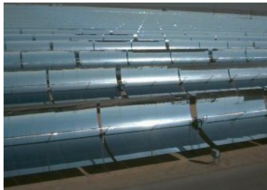
Parabolic Trough Power Plant
